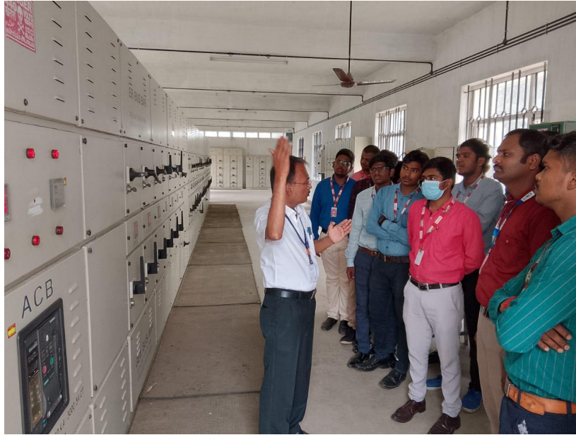
Figure 2 Busbar chamber in substation
