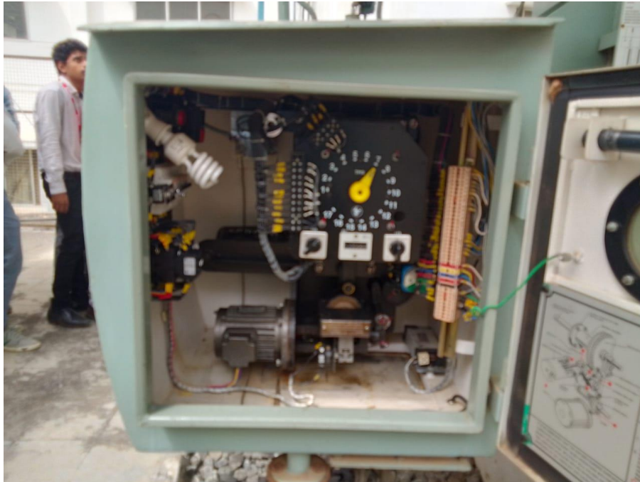
Figure 6 Onload Tap changer in transformer
