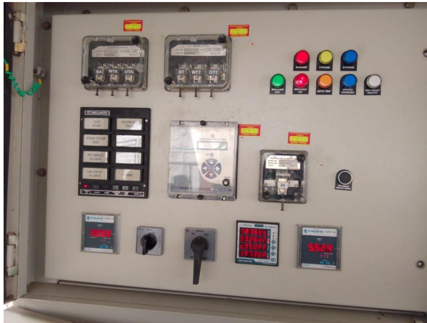
Figure 4 metering in substation
