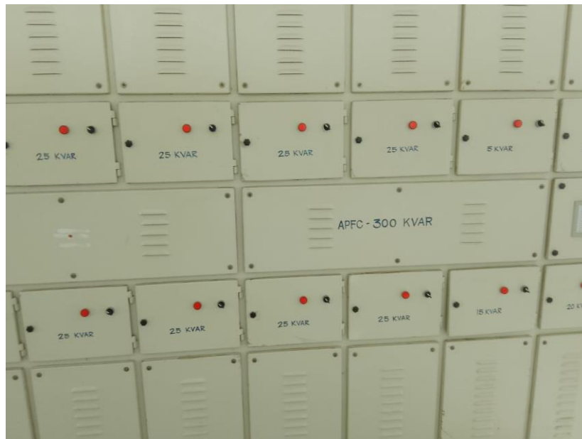
Figure 3 Automatic power factor correction
